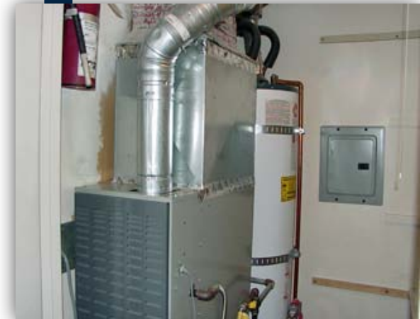
Individual Mechanical Room
